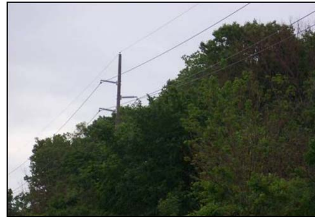
Vegetation growing into the lines
