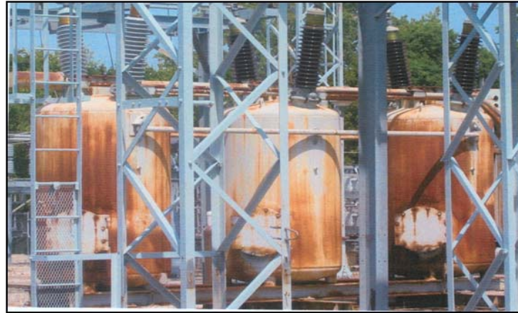
Breakers coated in rust
